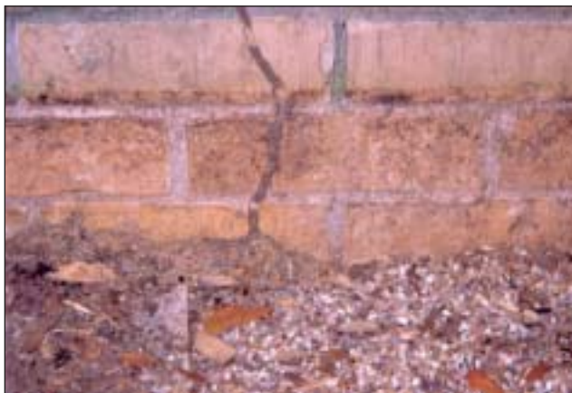
Figure 4a. Termite shelter tubes on foundation wall.
