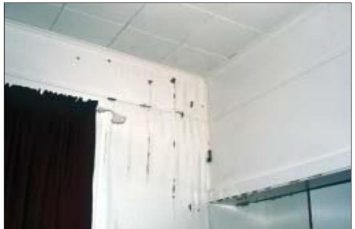
Figure 12. Shelter tubes on interior walls.
