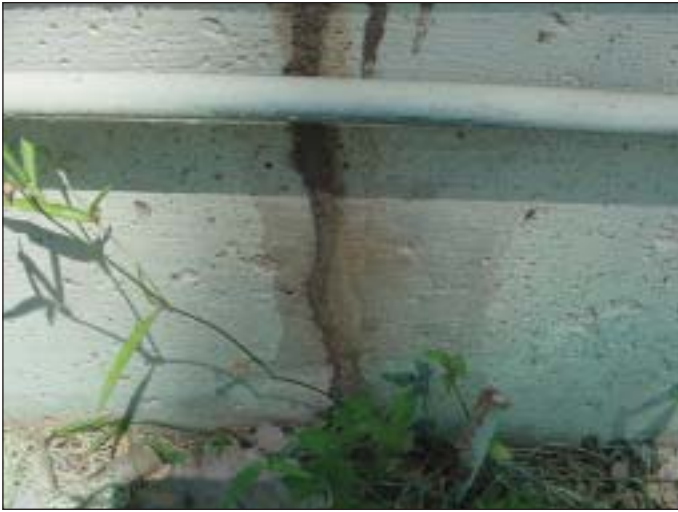
Figure 11. Shelter tube of an active termite colony.
