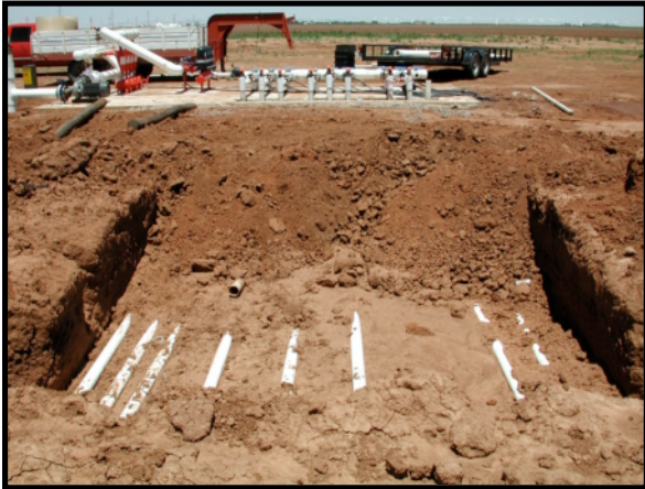
Figure 3. Zone lines going to SDI filter station, TAES, Helms, 2001.
