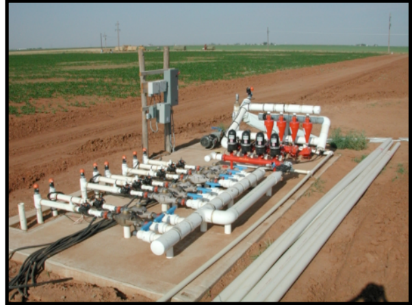
Figure 4. SDI filter station, TAES, Helms, 2001.
